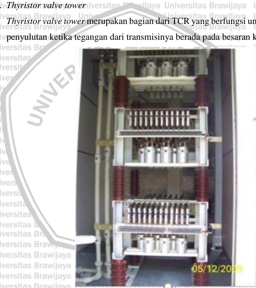
Gambar 2.13 Thyristor valve tower
