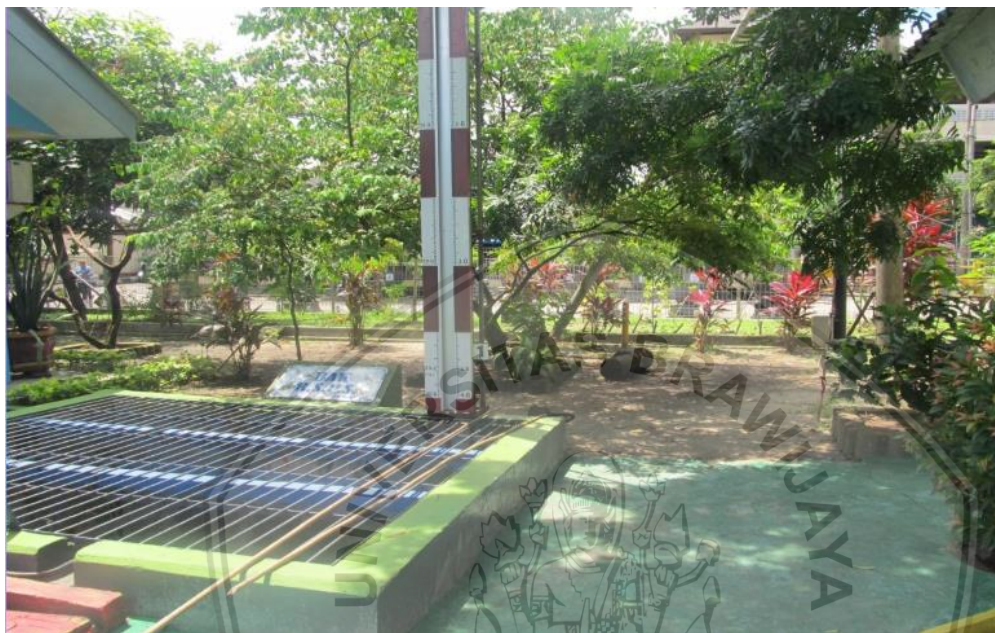
Gambar 4.32. Bak RSPS (Raw Sawage Pump Station) Sumber : dokumentasi pribadi
