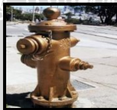
Gambar 2.15. Hydrant Sumber : www.hardwarestore.com
