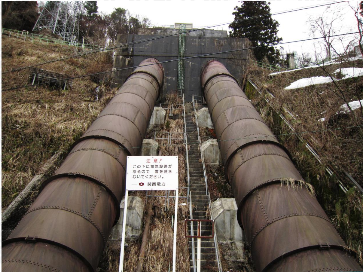
Penstock (pipa pesat)
