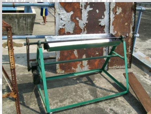
Gambar 3.2 Instalasi cylindrical parabolic collector
