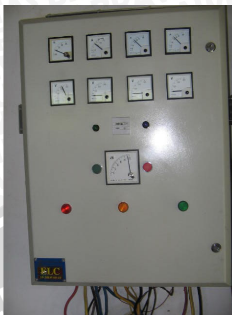
Gambar Load Contoller ELC GP Electronics STARCCTI bagian depan.
