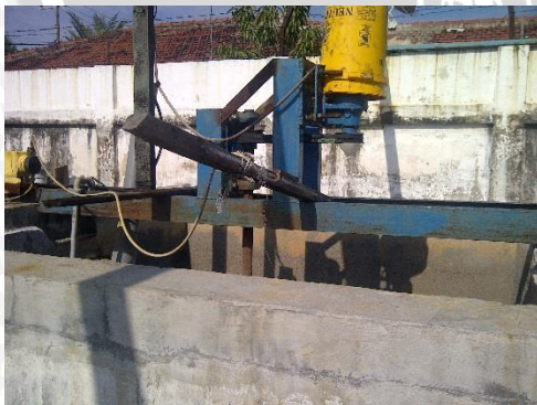
(IPAL pabrik asbes)
