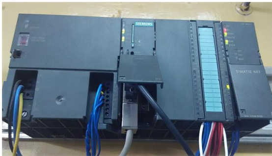
Gambar 2. 1 PLC SIMENS S7-300
