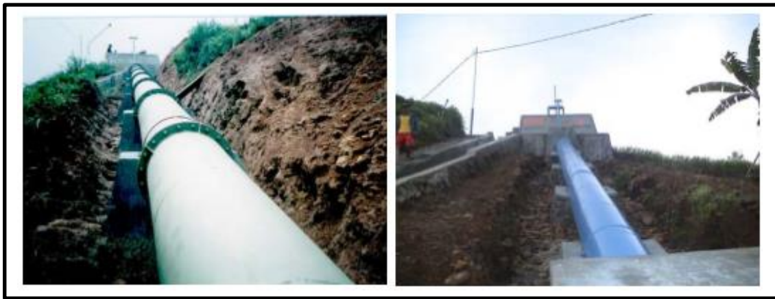
Gambar 2.45 Pipa Pesat ( Penstock ) Sumber: JICA (2009:2-4)
