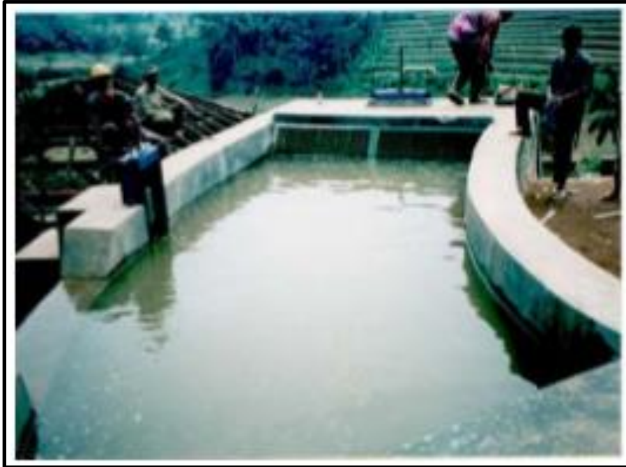
Gambar 2.42 Bak Penenang ( Head Tank ) Sumber: JICA (2009:2-4)
