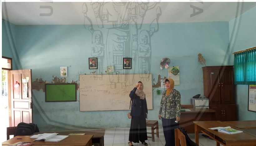
Figure 18. The broken walls condition in one of the classrooms at SDN Penatarsewu
