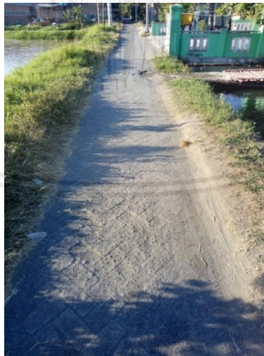
Figure 7. The paving road condition in Penatarsewu Village
