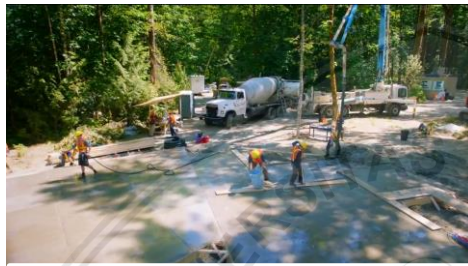
Figure 23: The land had been covered with cement.
