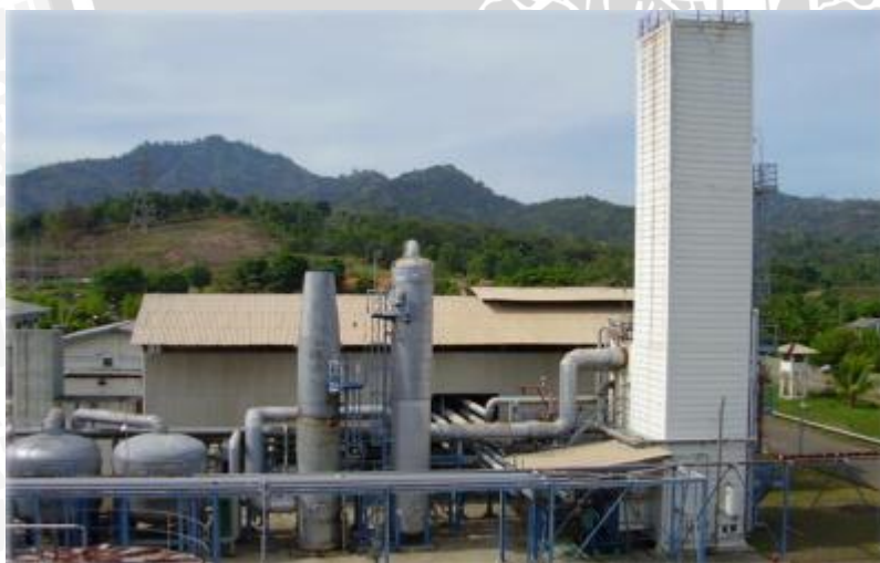
Gambar 4.2 Air Separation Unit Plant II Sumber : PT. Polychem Indonesia Tbk
