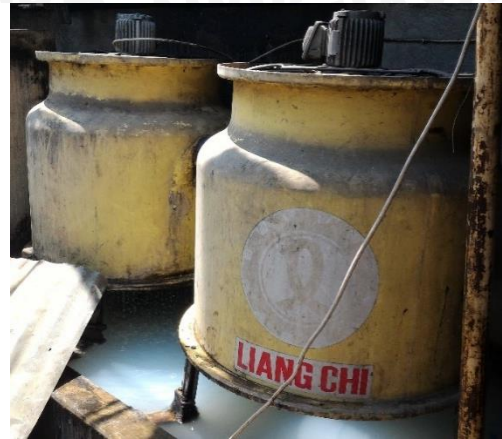
(b) Cooling Tower
