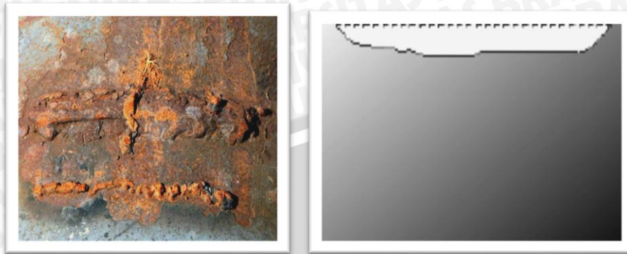
Gambar 2.13 Korosi merata ( uniform corrosion )
