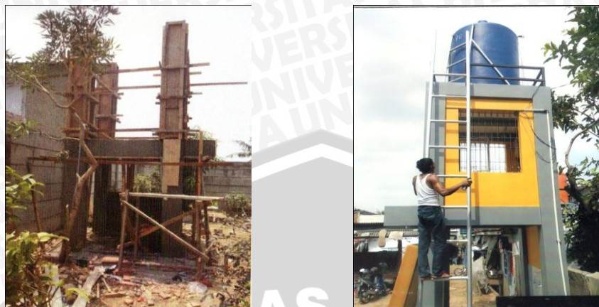
Figure 14. Water wells Construction in the Kelurahan Jatiuwung (Source: Documentation of Dinas PU Bidang Perumahan dan Permukiman Activities, 2012)
