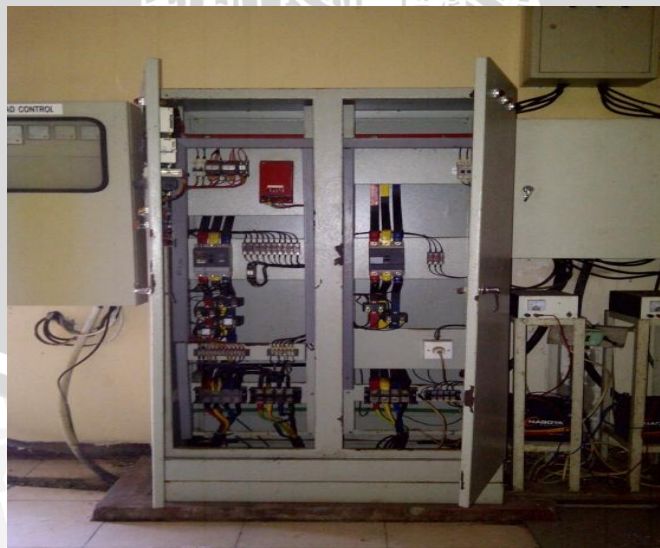
Gambar 13. Generator Distribution Panel
